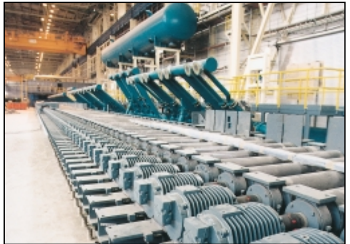
Application in the run-out roller table
