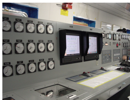
Engine Control Room
