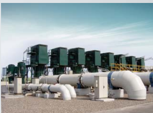
| Fujairah Desalination / UAE |
